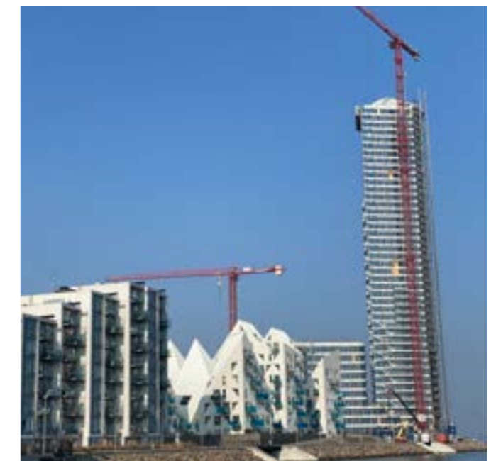
The Lighthouse currently under construction with The Iceberg development to the left
