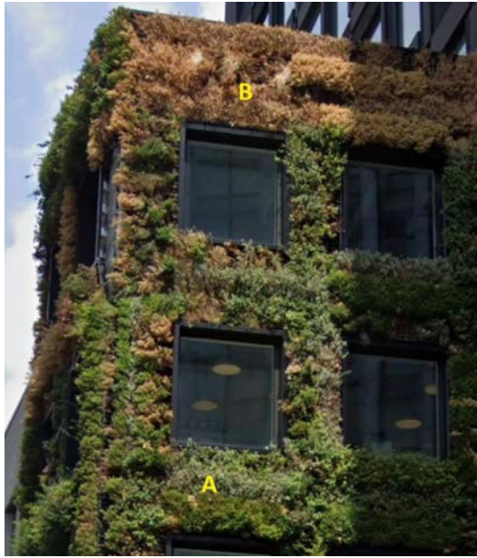
One example of a UK living wall installation with obvious variations in condition. The part marked at “B” is likely to fall well outside the condition of the lab tested samples and likely to surpass the minimum surface spread of flame requirement of ADB as it could be a class D or even an E!
