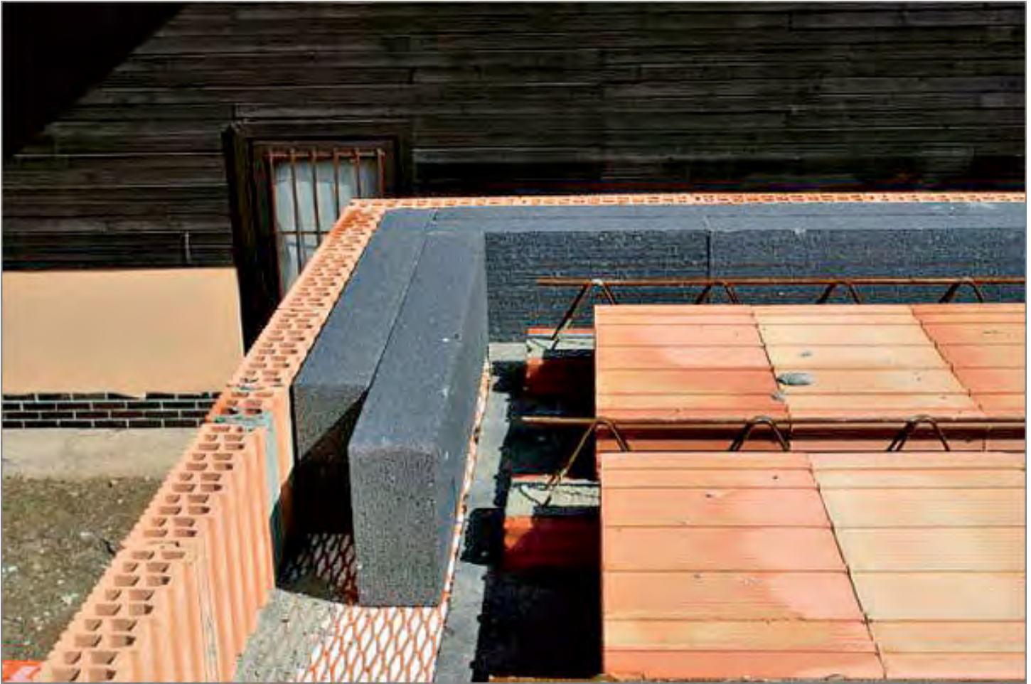
Preparing to cast a domestic floor slab using reinforced beams with ceramic/ clay blocks laid in between. Concrete is then cast onto the entire construction. This is a more manageable form of self shuttered block and plank construction.
