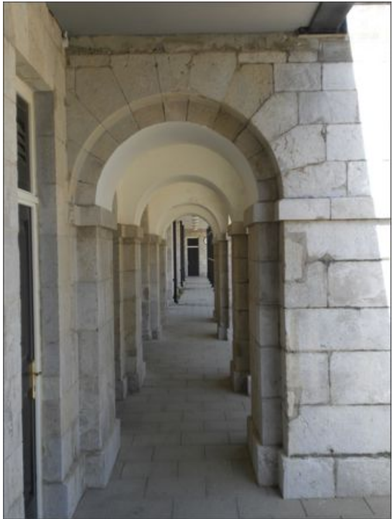
Former 1960 prefab corridor and office space demolished, with hidden lime stone exposed and restored.
