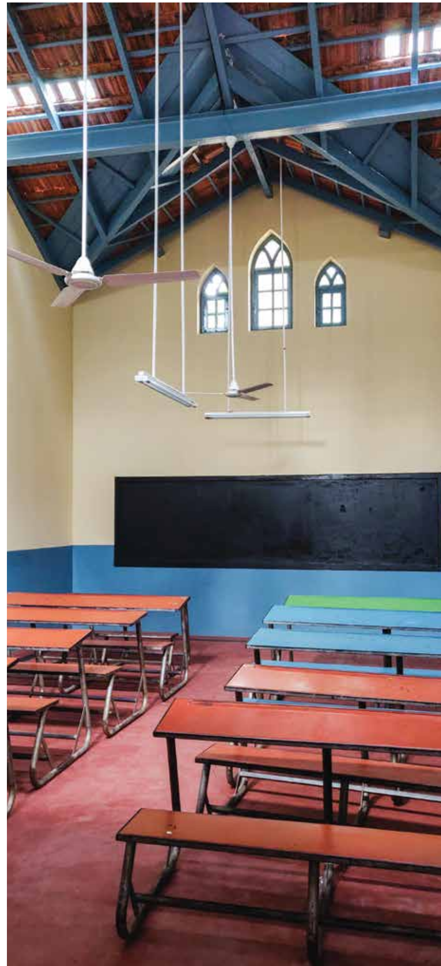
The damaged roof of the central hall before and after restoration. Above Photograph by Mahesh Chadaga
