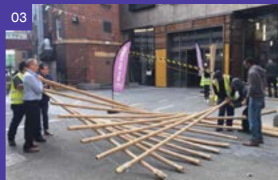
03 Laying the bamboo in grids and connecting the wires on the perimeter of the bamboo grid.
