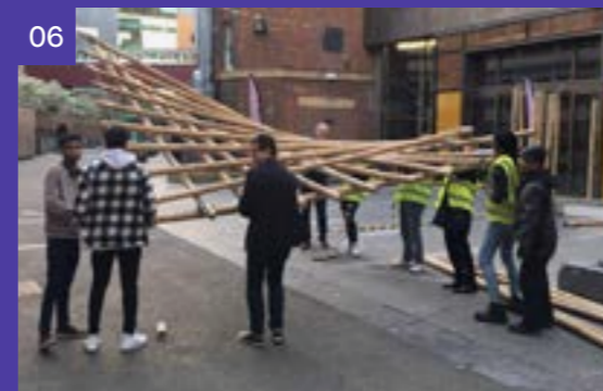
06 Moving the bamboo tensegrity roof onto a safe area for the next day construction under careful supervision of Dr Widyowijatnoko.
